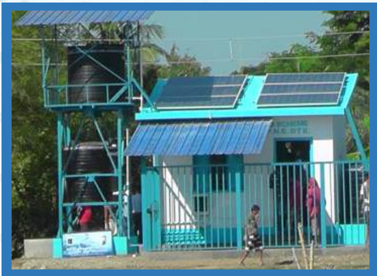
Step 5 th SOLAR PANELS (Supply Power to the Unit)
