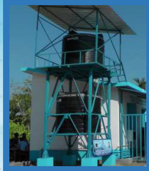
Step 3 rd TREATED WATER TANK (Upper Tank) INPUT WATER TANK UF (Lower Tank)
