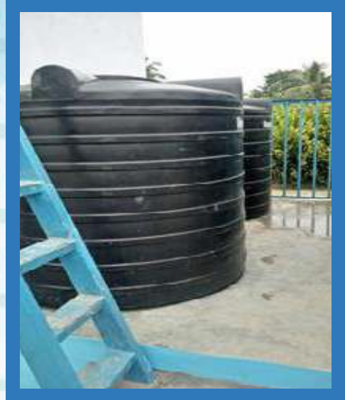
Step 1 st INLET TANKS 2 Nos (Connected in series) (Removes initial turbid load of raw water)
